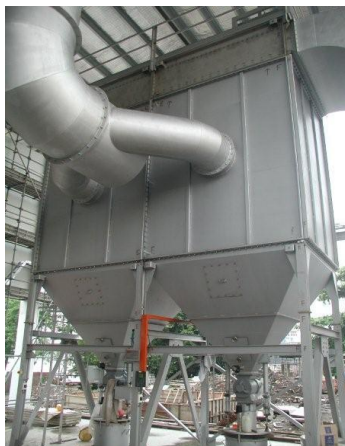
Fig. 5: a. Flue gases filter system.
