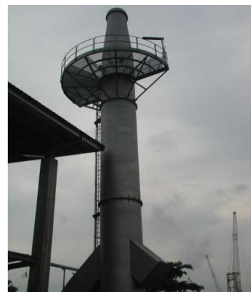
b. Exhaust chimney of flue gases
